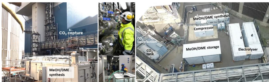
Fig. 5. left and middle - CO 2 capture pilot plant and synthesis plant at RWE's Innovation Center at Niederaussem, Germany. right - arrangement of the components needed for the CO 2 supply (compression, liquefaction and storage tank) and H 2 , (electrolyser) and synthesis plant with process gas compressor and storage site for the intermediates of the indirect route, methanol (MeOH) or dimethyl ether (DME).
